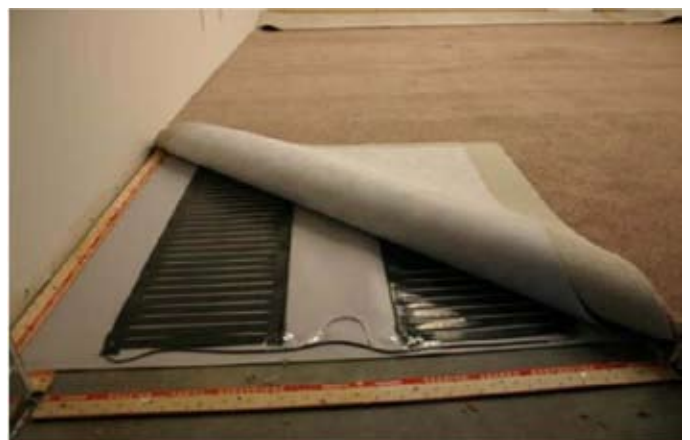
Elements on insulated concrete between two layers of carpet cushion and under carpet
